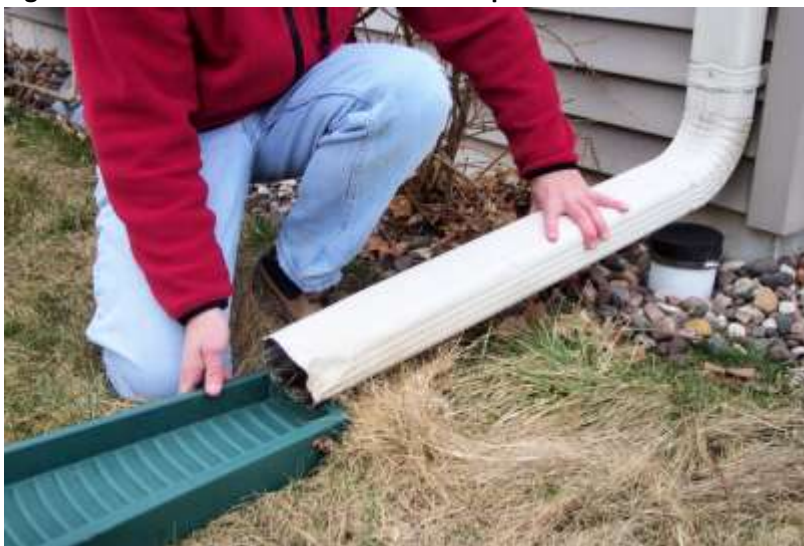
Figure 4-5 - Photo of Disconnected Downspout
