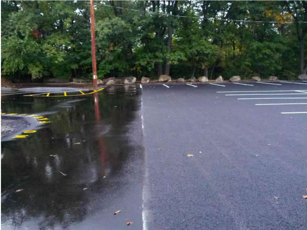
Figure 4-5 - Porous Asphalt Parking Lot
