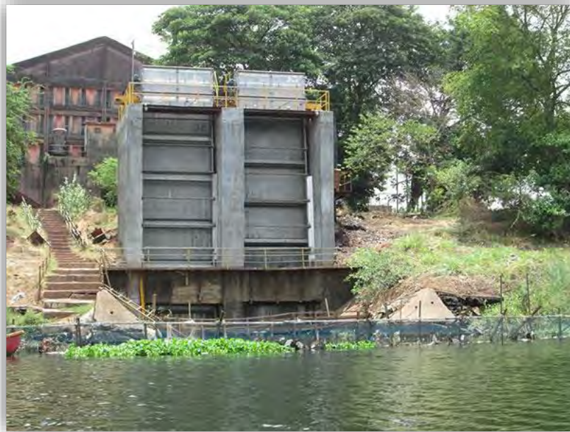
Photo No. 11 – Multi-Rake Mechanical Screen
