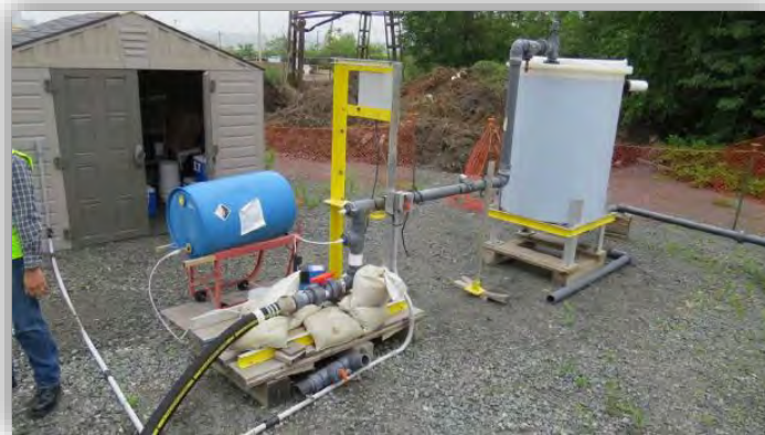
Photo No. 16 – Bayonne MUA Pilot Testing of Peracetic Acid
