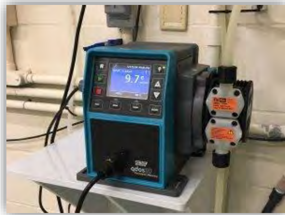
Photo No. 15 – Chemical Metering Pump
