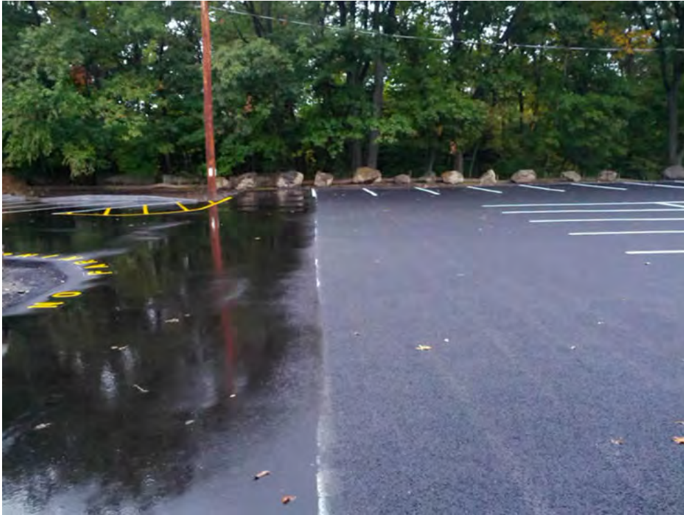
Figure 4-5 - Porous Asphalt Parking Lot
