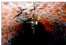
COMBINED SEWER SYSTEMS ARE OFTEN OVERSIZED AND IN NEED OF REPAIR
