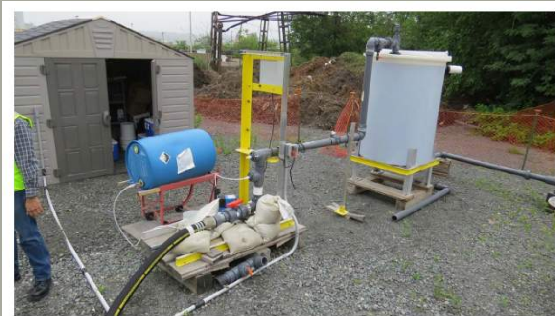
Figure 1. Peracetic acid Peragreen INJEXX system on project site
